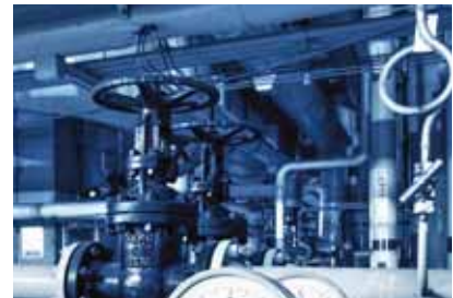
PIPING AND VALVES
